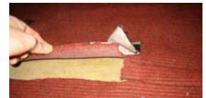
trip hazard on damaged carpet
