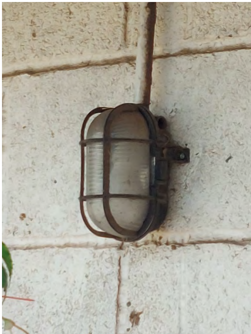
Fig. 2 - Exterior fitting – up to 7 fittings evenly spaced along the western wall; up to 7 fittings evenly spaced along eastern wall and two fittings on the southern (front) wall
