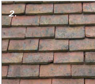
2. The most common roofing material is the red-brown clay tiles made from local Keuper Marl Clay. The clay tiles - called plain tiles - are of small scale, typically 265mm x 165mm, with a fine sand texture.
