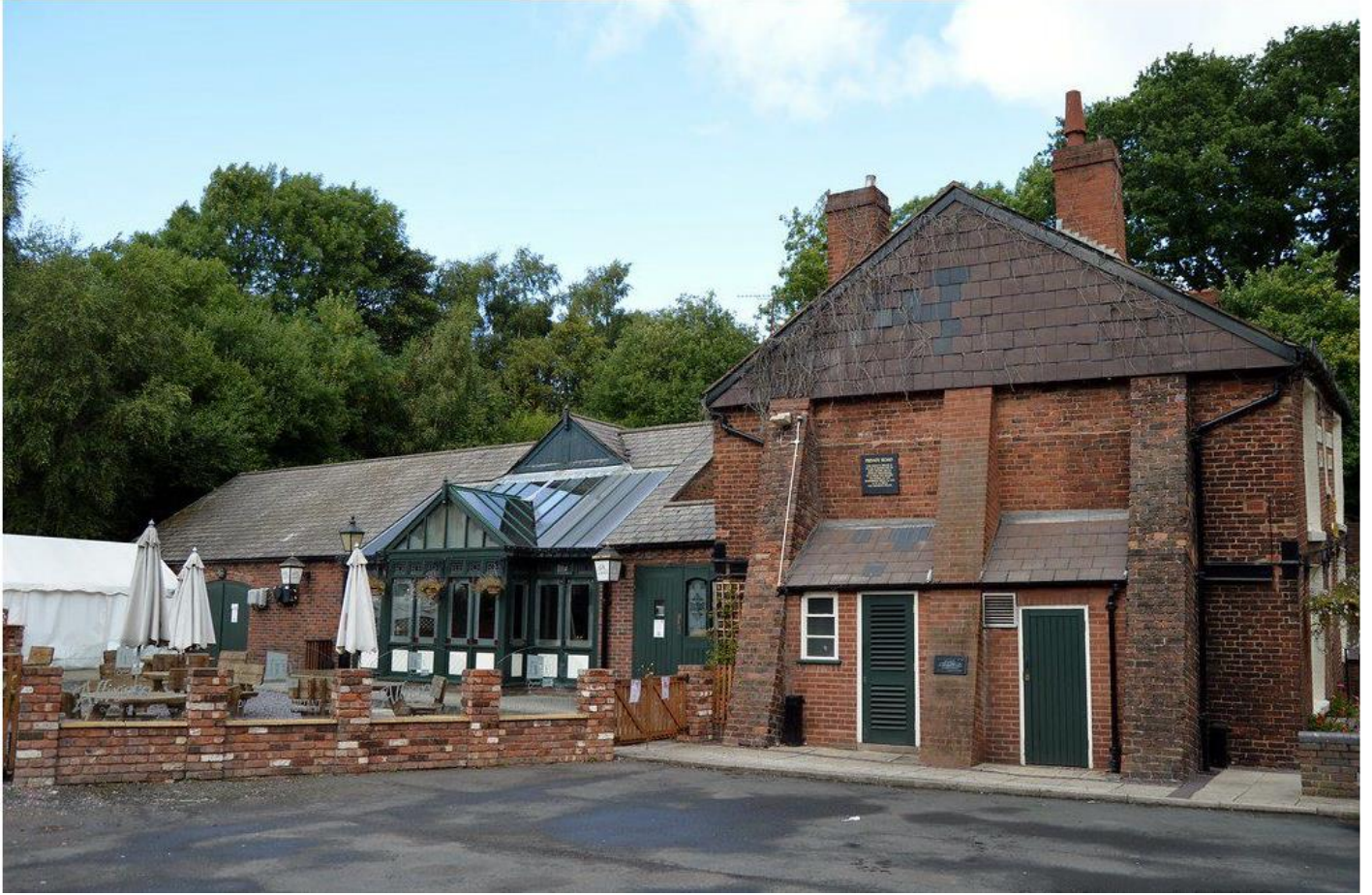
Detail view of the gable end of the 1765 building showing the three large buttresses and rear extension.
